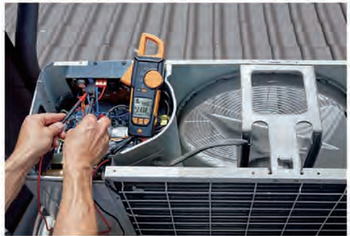
测量空调外机电压
